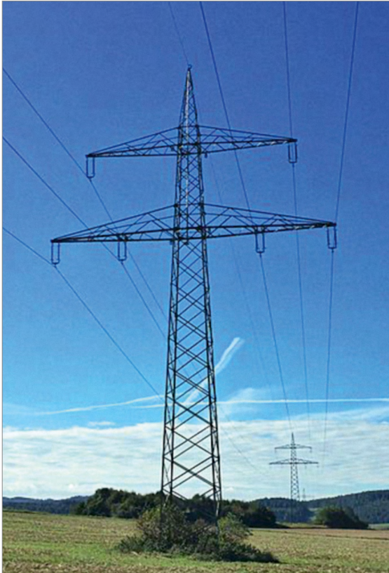
Figure 3.91: Danube pylon' with two 110 kV power circuits (left and right, each with three lines suspended from insulators) and earth wire on top of the pylon (source: Adl252, 110 kV Leitung Borken Lauterbach.jpg, CC BY-SA 4.0)
